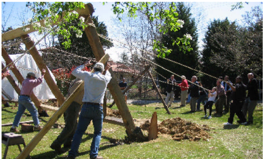
Russ Steele, Master Carpenter (foremost), guides the posts of the first wall of the Carpenter's Shop into place as many others raise the wall.
