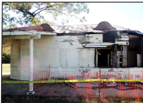
The Historic Concession Stand's Condition in 2013
