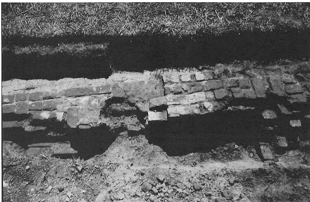
FIGURE 13. The interior of the west wall of the brick building showing the 6-foot wide interior firebox.
